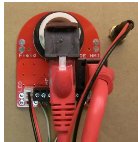
Figure 7 – MCC First - Field Panel Internal Arrangement
